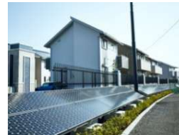
Community solar power generation system
